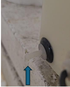
The fluid is slowly dripping out of the filter.
